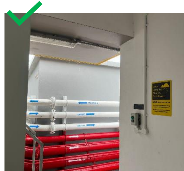
LPS warning sign
