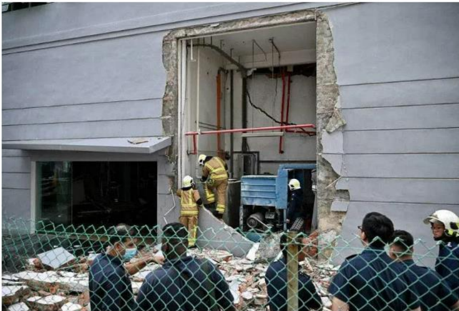
An explosion blew open a section of the Audi service centre in Ubi on March 7, 2023. ST PHOTO: KUA CHEE SIONG
