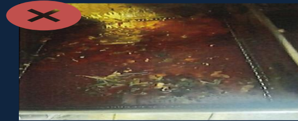
Badly maintained grease interceptor
