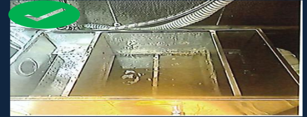
Well-maintained grease interceptor with clear last compartment
