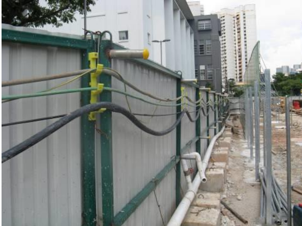
Proper cable hangers use to hang up cables
