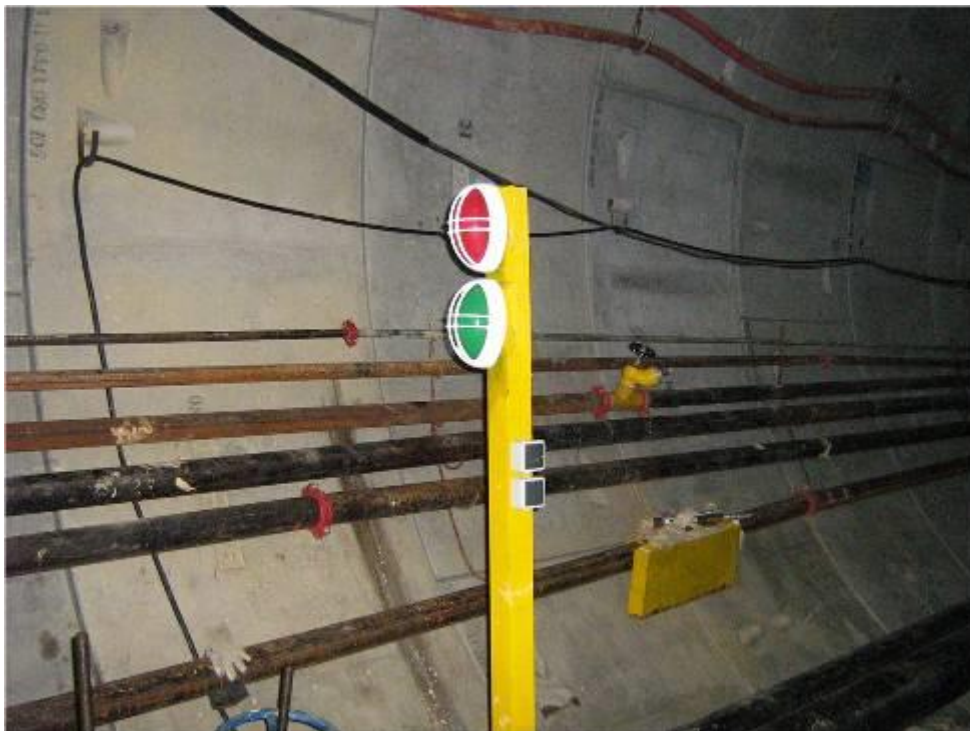
Red and Green signal light to regulate locomotive movement in the tunnel
