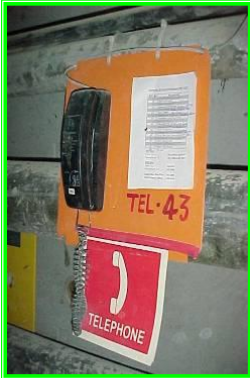
Telephone provided at regular interval along tunnel to notify of any emergency
