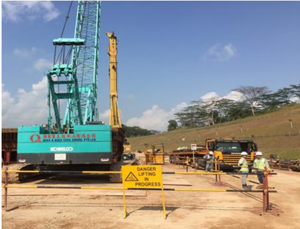
Lifting activity is cordoned off and warning signage is placed to warn personnel against entering the area
