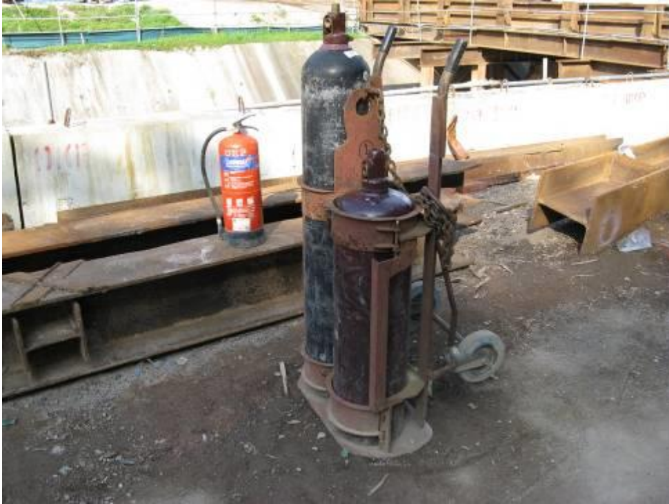
Gas cylinders secured in a cylinder trolley to prevent toppling
