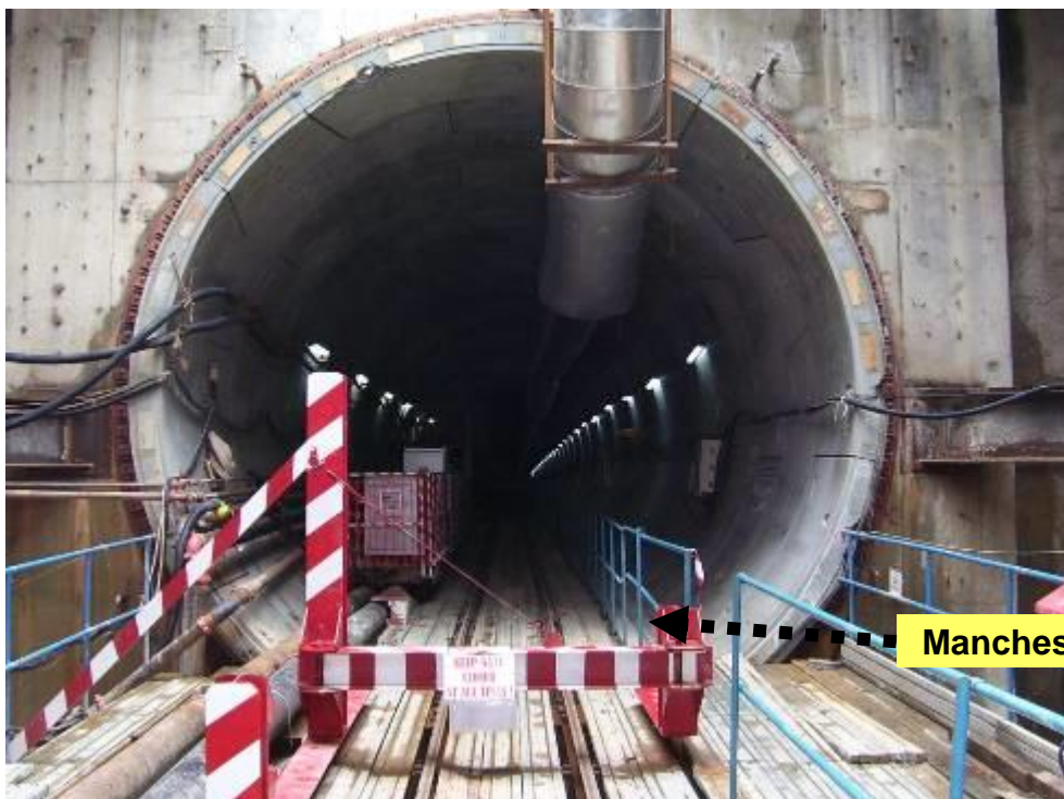
Manchester gate installed to regulate movement of locomotive in tunnel
