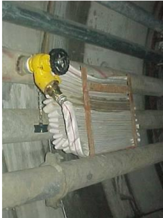
Fire hose reel provided at regular interval along tunnel for fire fighting purpose
