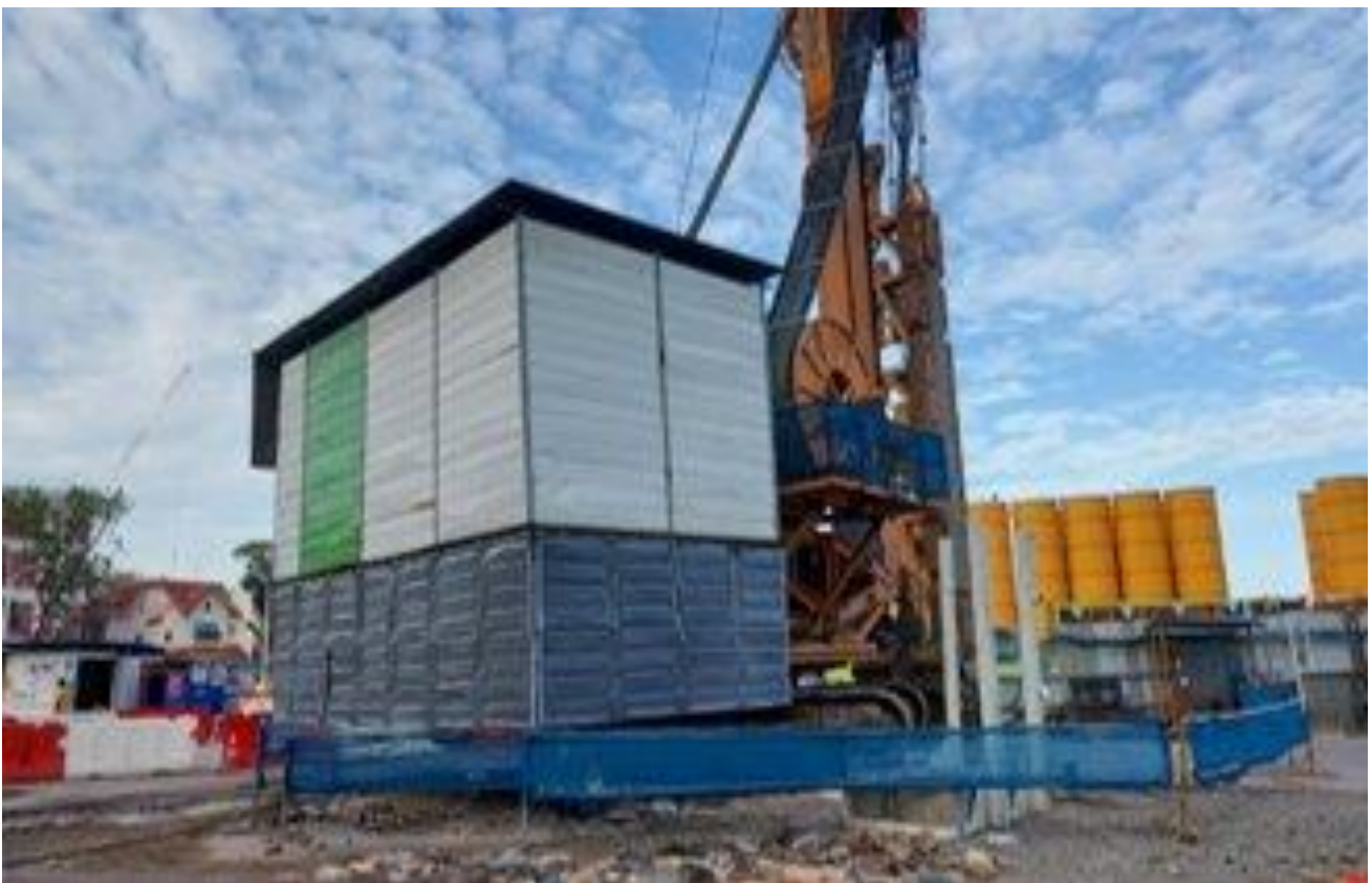
Use of localised noise barriers for noisy machinery (eg. Diaphragm Wall Cutter)
