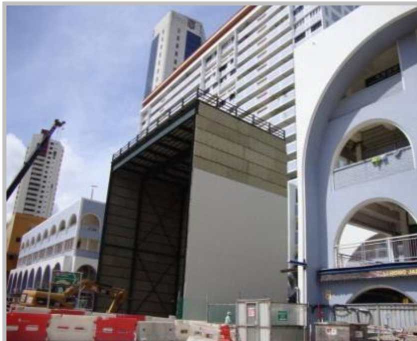
Large acoustic enclosures used for noisy activities / machineries (For e.g. excavation activities, launch shaft) conducted near noise sensitive receivers)
