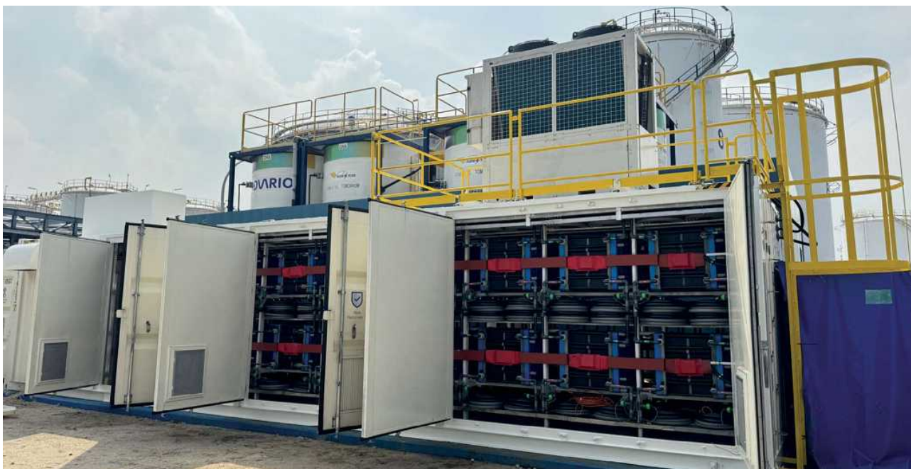
VFlowTech was selected to pilot the first vanadium redox flow battery (VRFB) using existing storage tank infrastructure, with electrolytes produced from recycled industrial waste to enhance circularity, supported by Energy Market Authority (EMA), JTC, and Enterprise Singapore under a clean energy innovation grant. The 400 kW/1,600 kWh (1.6MWh) VRFB is located at Advorio's site on Jurong Island.
