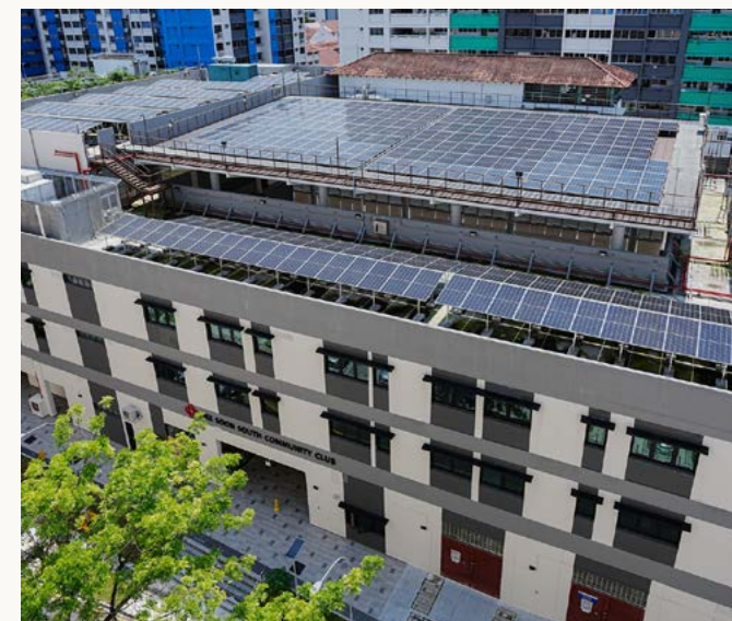
Solar panels on the roof of Nee Soon South CC.
