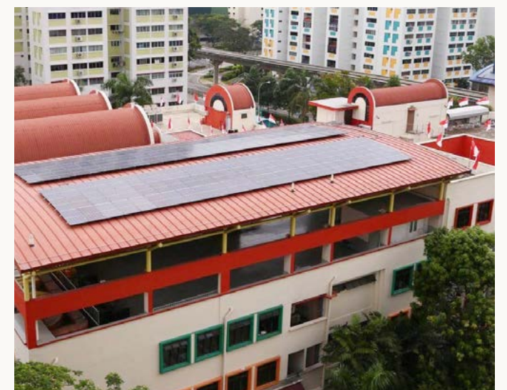
Changi Simei CC (top) and Bukit Panjang CC (below) are two key PA buildings that have solar panels installed on the rooftops.
