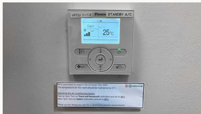
Air-conditioning temperature control at 25 degrees Celsius at PAHQ.
