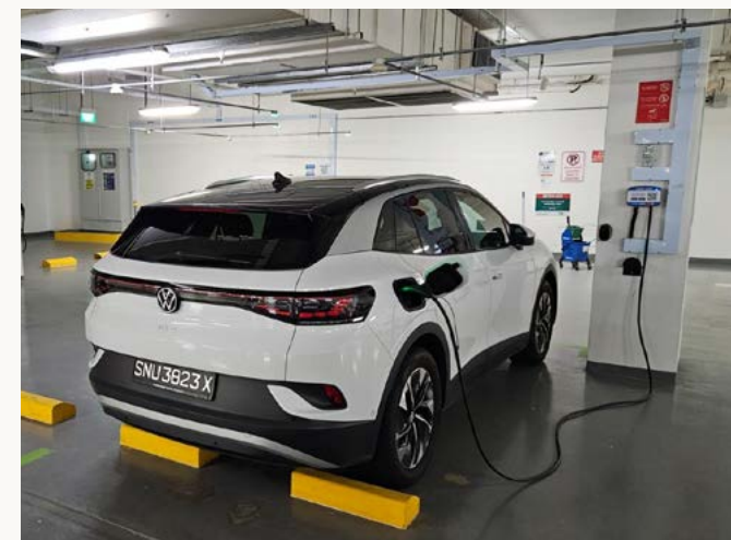
EV charging station at a PA facility.
