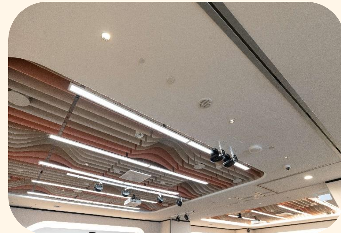
Acoustic Panels and Tracks for Operable Walls
