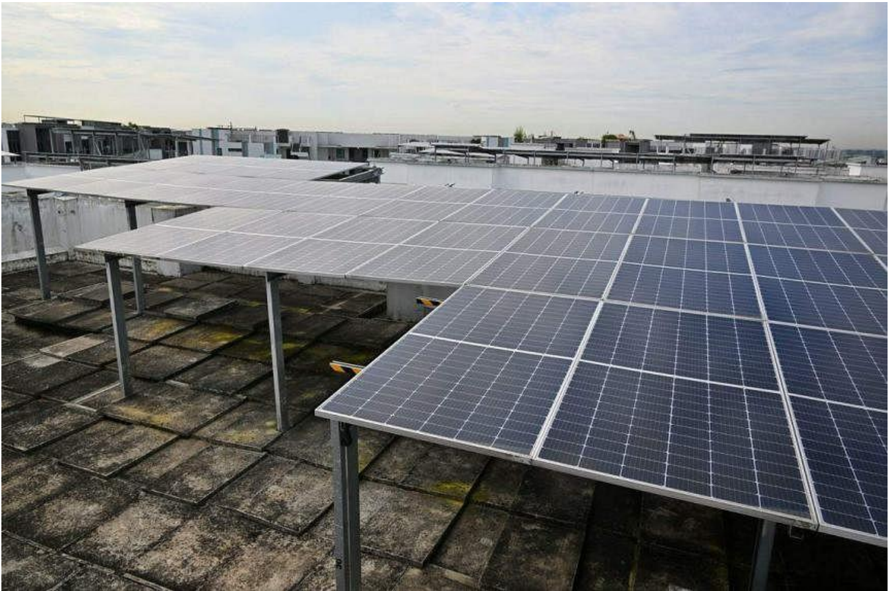
Some of the ways to cut emissions is to harness electricity from green energy sources. ST PHOTO: CHONG JUN LIANG
